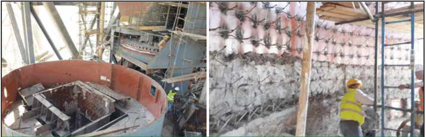
HOTDISC installed on Line 1
