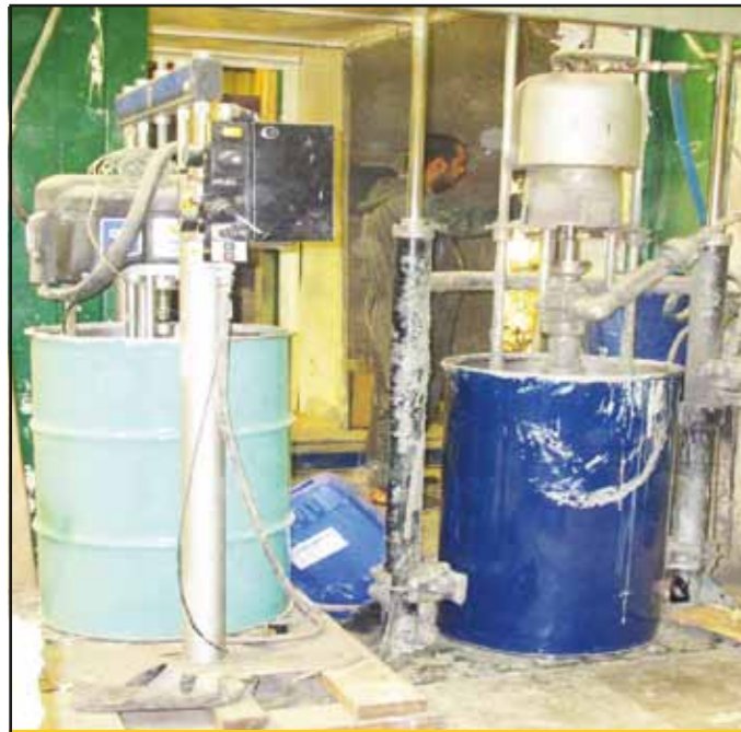
Before: Chemical feeding system
