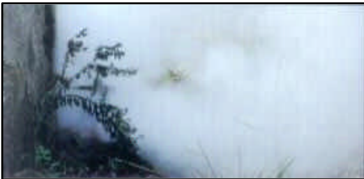
Steam leaking from defective steam traps
