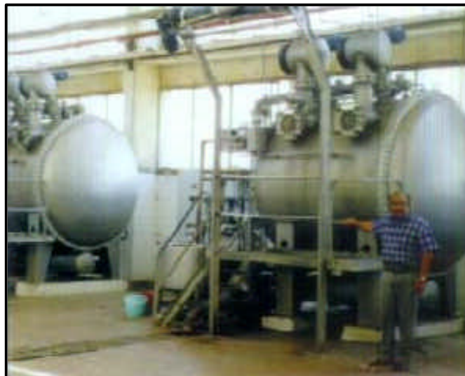
Jet machines at Dakahleya used in Sulphur Black dyeing
