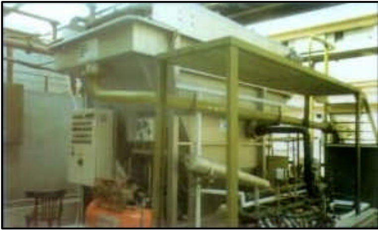
Dissolved Air Flotation Unit installed in Tanta Factory
