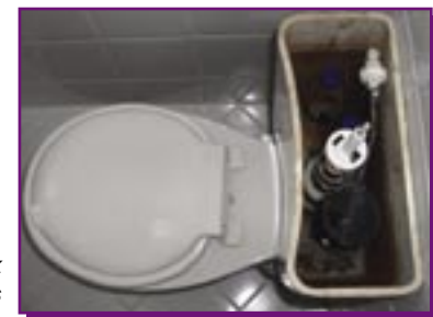
Reducing flush tank capacity in toilets
