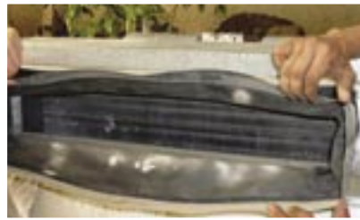
Air conditioning unit with rivets
