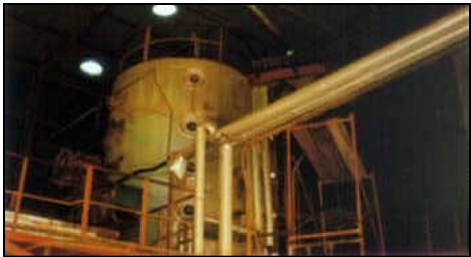
Insulation of steam pipes and steam network upgrading reduced energy costs by 48%
