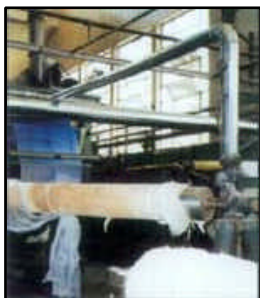
Steam pipe insulation in the factory has saved LE135,126 per year
