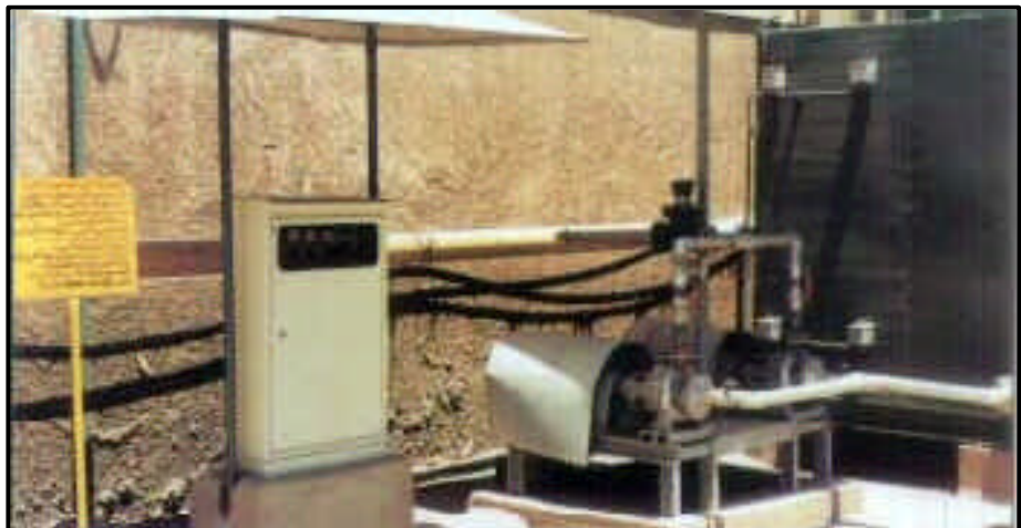
Installed condensate recovery system comprising collection tank, pumps, flow meter and control panel. Annual savings are LE135,100
